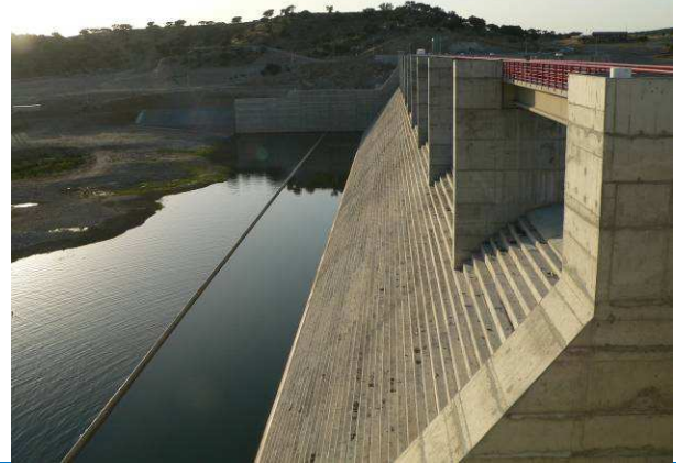
Pedrogão dam (Portugal) A RCC gravity dam (H = 43 m, L = 473 m) with uncontrolled stepped spillway
